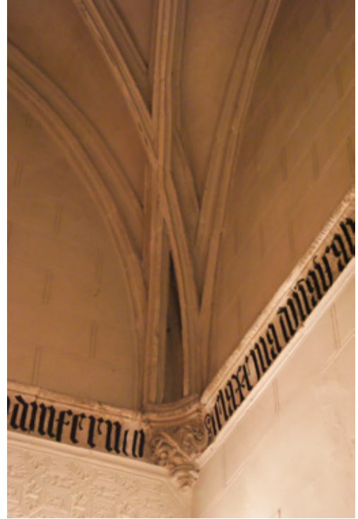
Fig. 4. Corbel and vault ribs, south west corner, Candelaria chapel, church of San Justo y Pastor, Toledo. Chapel completed by 1497. Source: Costanza Beltrami
